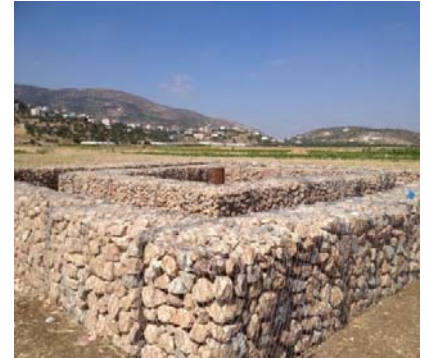
Figure 4: Filtration System - Gabions
